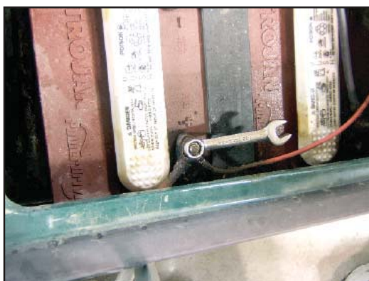
24. Positive Battery Connection
